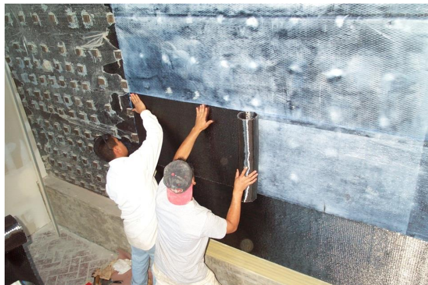
Figure 57: Strengthening of a 'shear wall' (reinforcement wall that is widely used in earthquake-sensitive structures) with carbon-composite [5]
